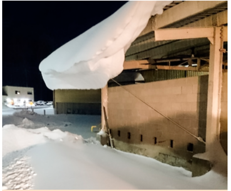
Snow overhangs a shed next to the warehouse.
