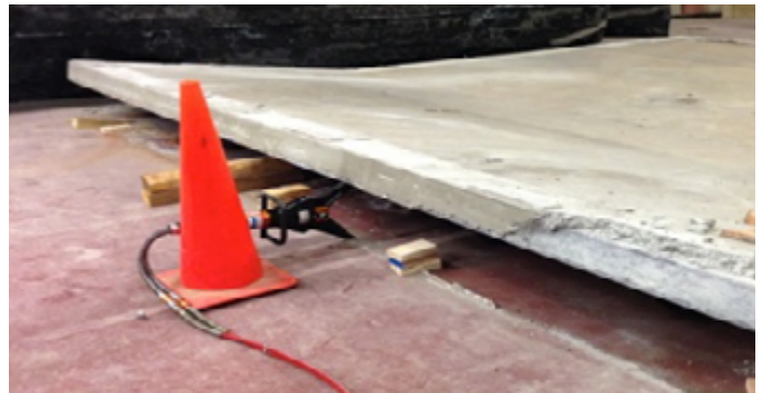
The concrete slab after it was successfully lifted off the ground. (Photo by Steve DePasquale)
