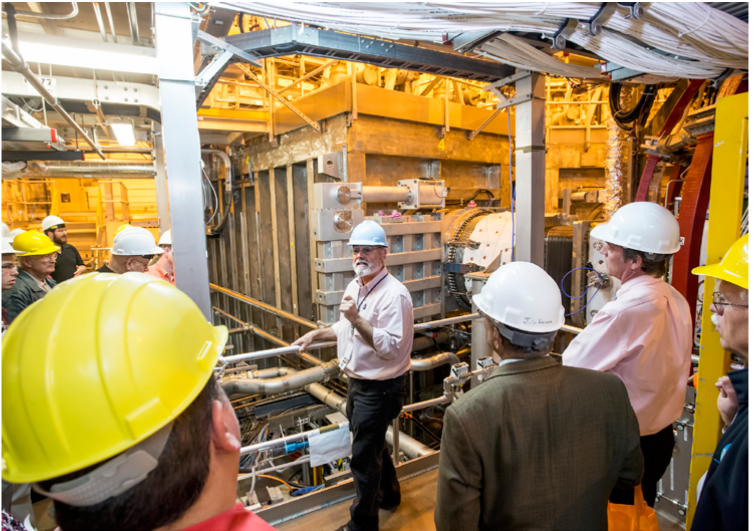
Al von Halle shows the second neutral beam injector in the NSTX-U test cell.
