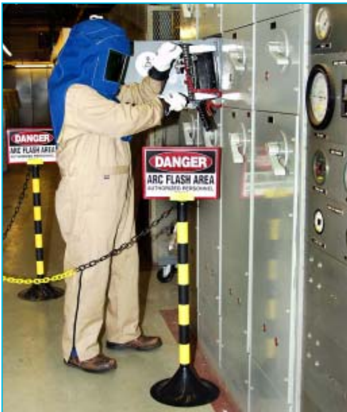
Art Wise in protective clothing and gear as he inserts a starter bucket into a Motor Control Center.
