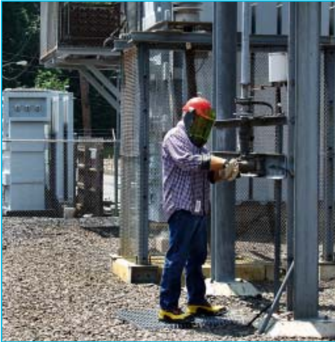
Dick DeBonis in protective clothing and gear as he operates a gang operated 138 kV disconnect switch.
