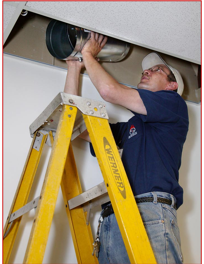
Kevin Taylor of Master Fire Protection installs a damper for the Variable Air Volume Air Handling Unit upgrade in a Lyman Spitzer Building office. When the project is completed, 87 zones will have new units, leading to greater energy efficiency.
