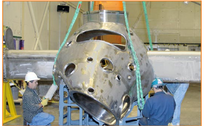
Staff, using a crane and rigging, place the vacuum vessel segment in the NCSX Coil Winding Facility.
