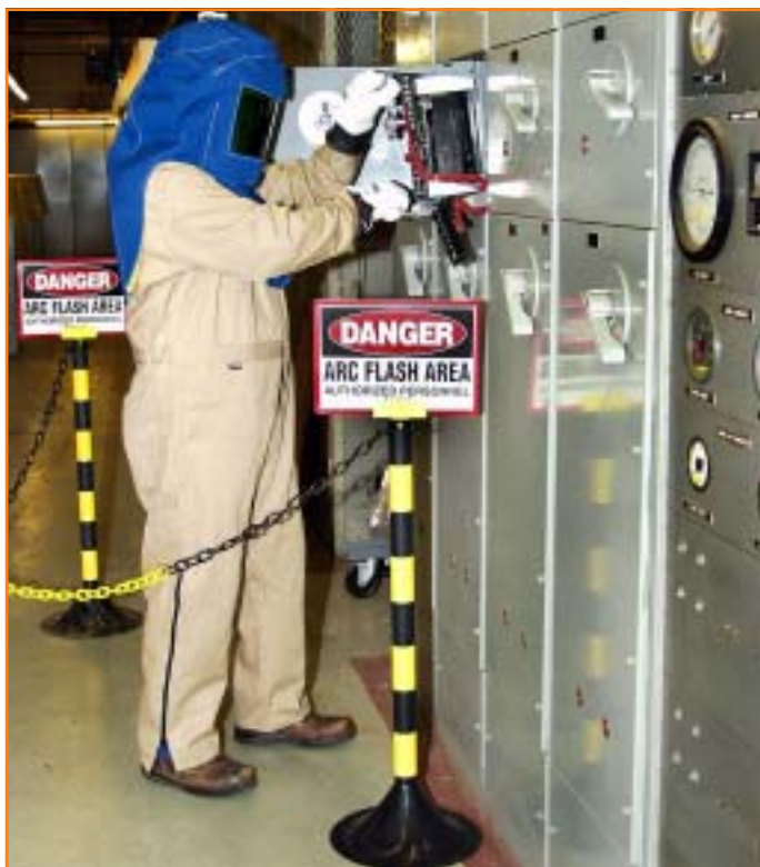
PPPL's Art Wise in protective clothing and gear as he inserts a starter bucket into a Motor Control Center at the Lab.
