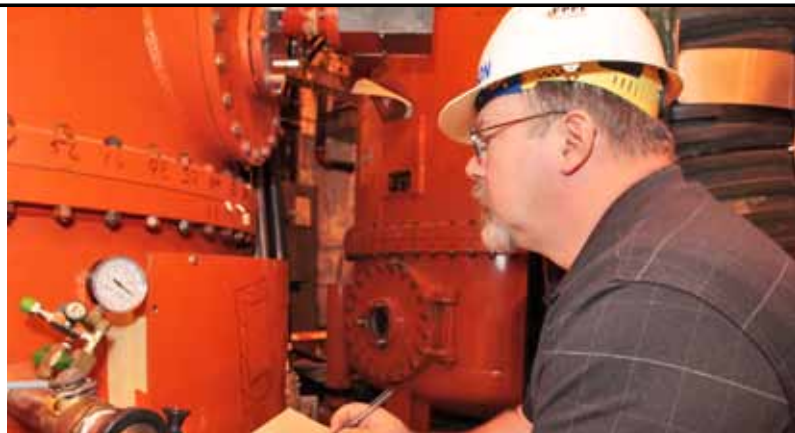
Tim Stevenson takes inventory of SF 6 levels at a power supply tank for one of PPPL's experiments.
