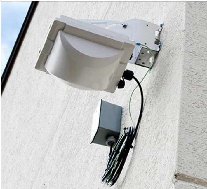
One of the outdoor antennas. The antennas are waterproof and have their own heating systems to operate in any weather.
