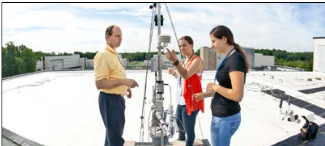
Keith Rule and a team of interns felt the heat when they installed a weather station on top of the LSB roof last summer as part of the cool roofs project. From left to right: Keith Rule; Jessica Sponaugle, a summer intern from Monmouth University in West Long Branch; and Hannah Capponi, a summer intern from Council Rock High School North in Newtown, Pa.
