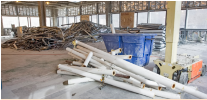
Piles of sorted debris on the LSB Annex third floor will be carted away and recycled.
