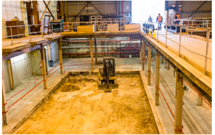
One of the two tractors that will dig holes for footers to install columns in the C-Site MG Building.
