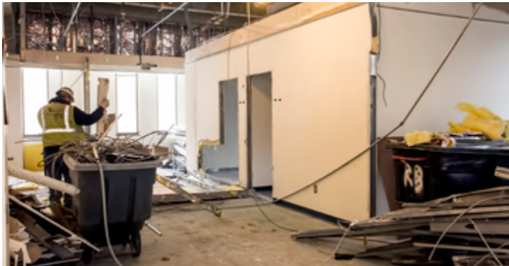
The demolition of the second floor of the LSB Annex is still in progress.
