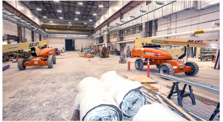
Most of the work has been completed on the C Site MG Building. (Photo by Elle Starkman)
