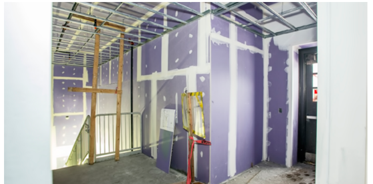
The walls of the building have been sheetrocked and a few areas still need painting. (Photo by Elle Starkman)
