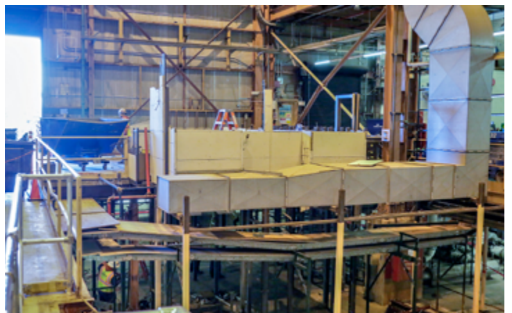
A metal structure on the first floor of the MG building is being disassembled. (Photo by Elle Starkman)
