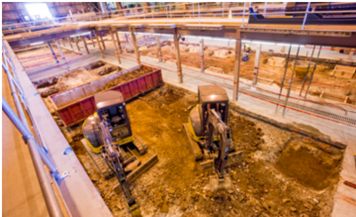
A bulldozer and jackhammer dig holes in the soil in the C Site-MG building basement. (Photo by Elle Starkman)
