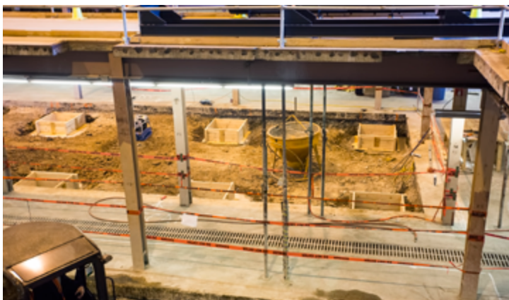
Wooden frames for the concrete foundations of steel pillars that will hold up the cement slab filling in the first floor. (Photo by Elle Starkman)
