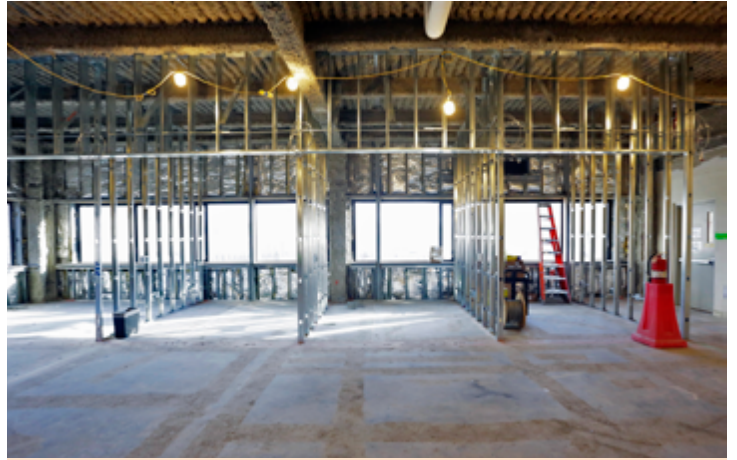
Metal frames of offices on the third floor of the Lyman Spitzer Building Annex. (Photo by Elle Starkman)
