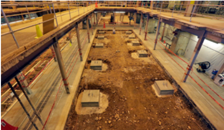
Cement footers in the basement of the C Site-MG Building. (Photo by Elle Starkman)
