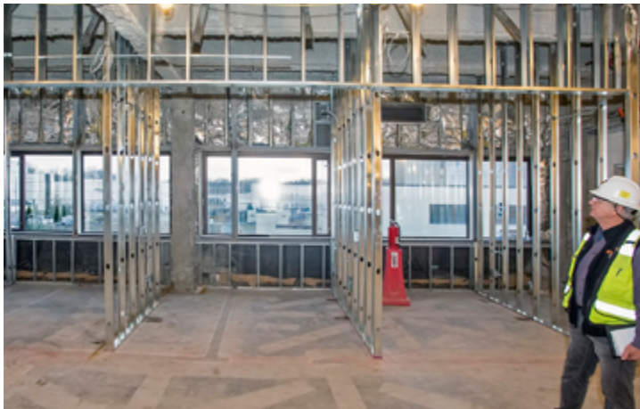
Frank Karam, the Princeton University field engineer for PPPL's Infrastructure Operational Improvements (IOI) project, examines metal studs for offices in the Lyman Spitzer Building Annex. (Photo by Elle Starkman)
