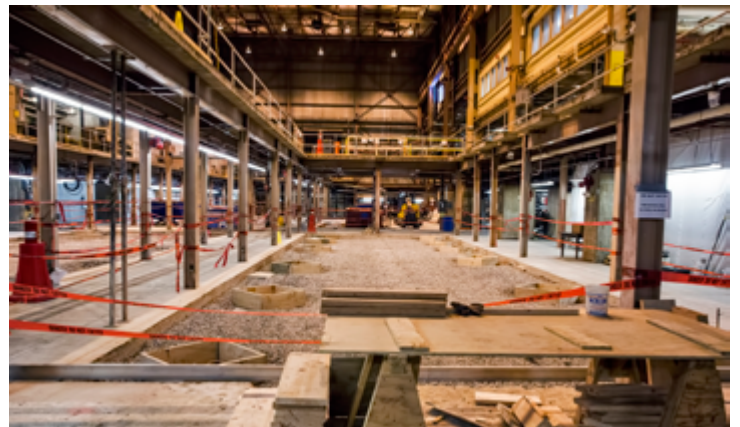
Crushed stone has been laid out in the basement and footers are ready for steel pillars to support the cement slab floor on the first floor. (Photo by Elle Starkman)
