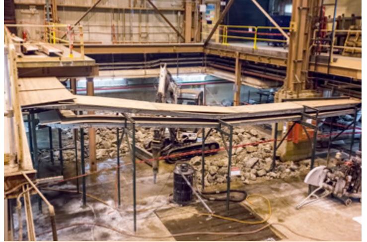
A jackhammer was used to break up the concrete floor in one corner of the MG Building. (Photo by Elle Starkman)
