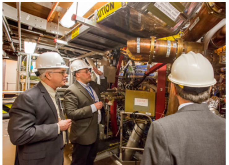
Jonathan Menard, center, shows Peurrung, left, and Michael Zarnstorff, right, the NSTX-U test cell. (Photo by Elle Starkman)
