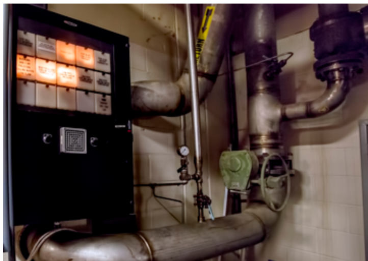
A cooling water system alarm panel at D Site. (Photo by Elle Starkman)
