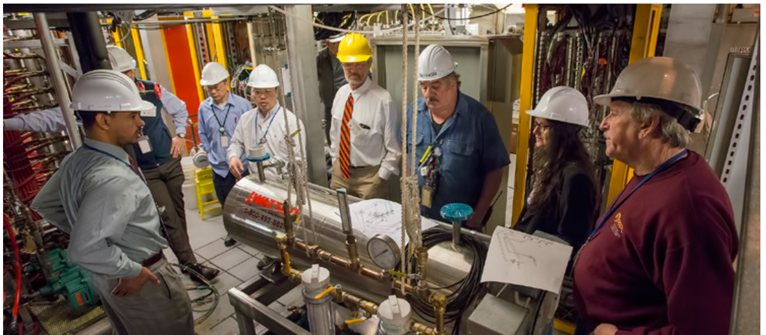
Neway Atnafu, left, the DVVR committee and other PPPL engineers and technicians involved with the review look at a new OH water heater, at right, which will soon be installed. From left: Stefan Gerhardt, deputy head of engineering for the NSTX-U Recovery Project; engineers Feng Cai and Danny Cai, Geoffrey Gettelfinger, department manager of the Physics Department at Princeton University and a former PPPL engineer; technician John Desandro; Valeria Riccardo, head of engineering; and engineer Pete Titus. (Photo by Elle Starkman)
