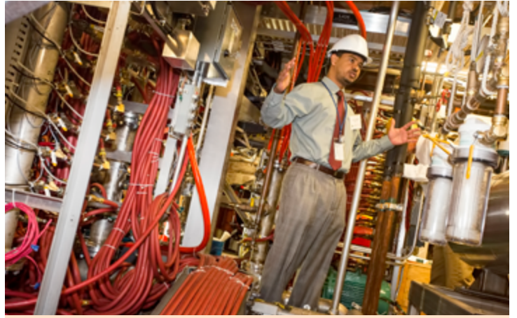
Neway Atnafu shows the tour group the water cooling system connected to the NSTX-U. (Photo by Elle Starkman)
