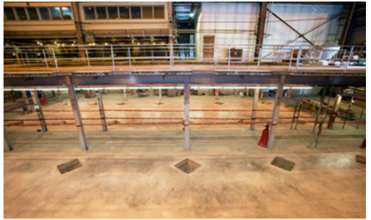
Steel pillars will be installed in the concrete floor of the C Site-Motor Generator Building. (Photo by Elle Starkman)
