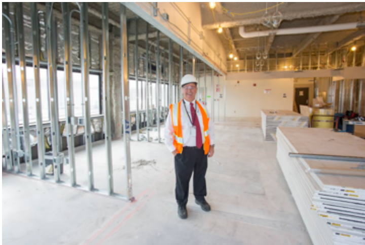
Les Hill, head of the IOI project, stands next to piles of sheetrock on the third floor of the LSB Annex. (Photo by Elle Starkman)
