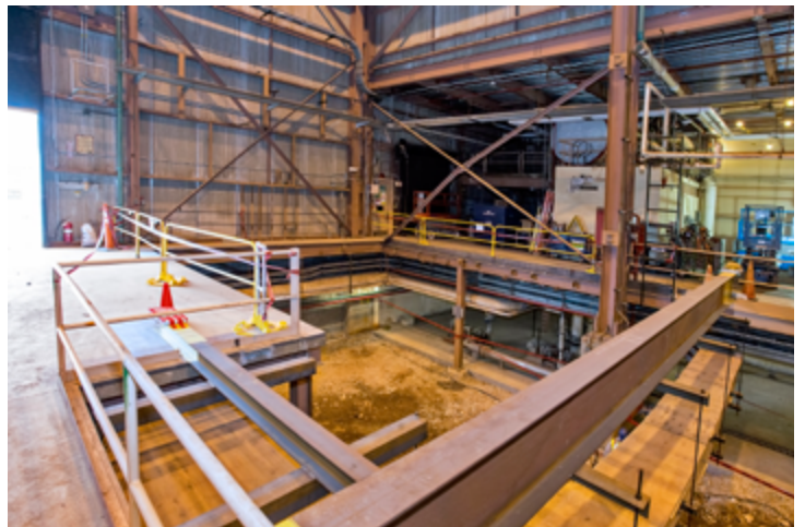
The southeast corner of the building is still being excavated. (Photo by Elle Starkman)
