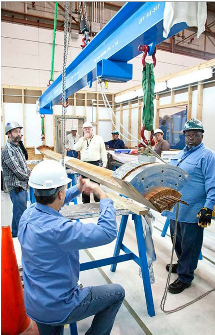
Guided into position: The completed first quadrant is moved into place to await the remaining three sections of toroidal field conductors that will join it in the NSTX-U center stack.
