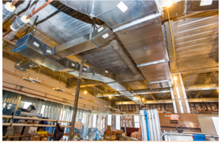
Ductwork is being installed on the first floor of the Lyman Spitzer Building Annex. (Photo by Elle Starkman)
