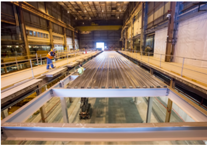
Metal decking will be the base for a concrete deck on the first floor of the C Site-MG Building. (Photo by Elle Starkman)
