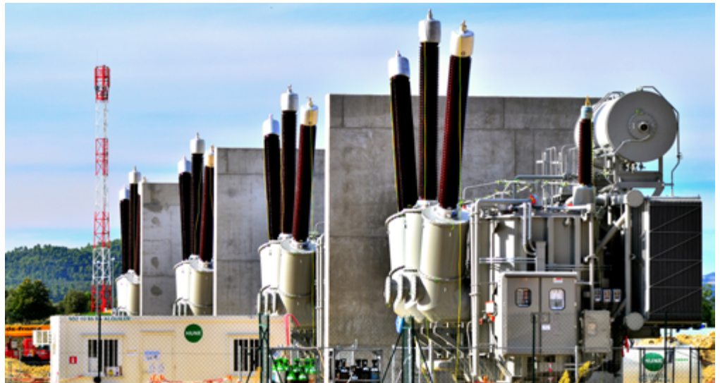
The transformers at ITER. (Photo courtesy of Fusion 4 Energy)
