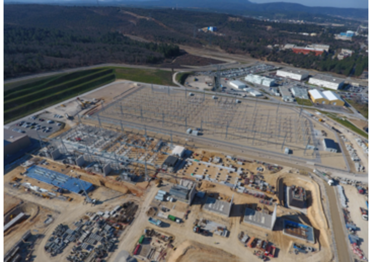
An overhead shot of the ITER switchyard. (Photo courtesy of ITER)
