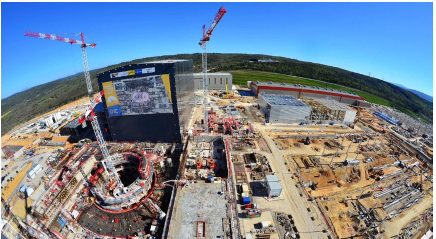
An aerial view of the ITER site taken in April. (Photo courtesy of ITER)
