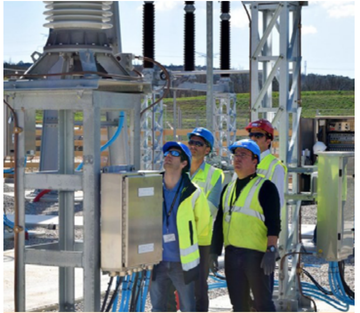
From left, Jeremy Sanna (ITER Organization), Cedric Gazza (ENGAGE), Gilles Consolo (ITER Organization operation manager for the 400kV switchyard) and Laureano Linan Delgado (FERROVIAL) verify the 400 kV circuit breaker before commissioning. (Photo Francesco Campostrini/ITER Newslines)
