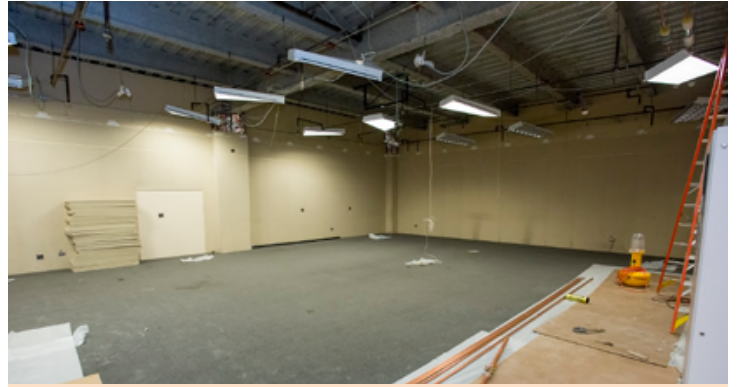
Contractors will install new HVAC systems in the ceiling of the Control Room Annex. (Photo by Elle Starkman)
