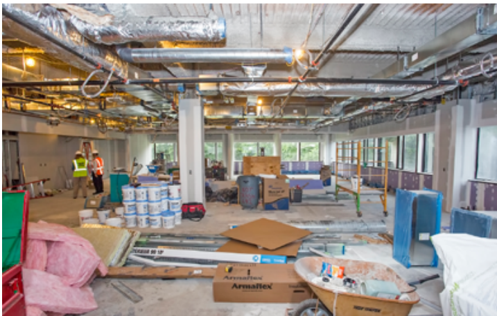
Progress on the walls of the 2nd floor of the LSB Annex. (Photo by Elle Starkman)
