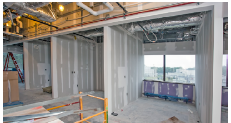
Sheet rock and spackling for office walls on the first floor of the LSB Annex is progressing. (Photo by Elle Starkman)
