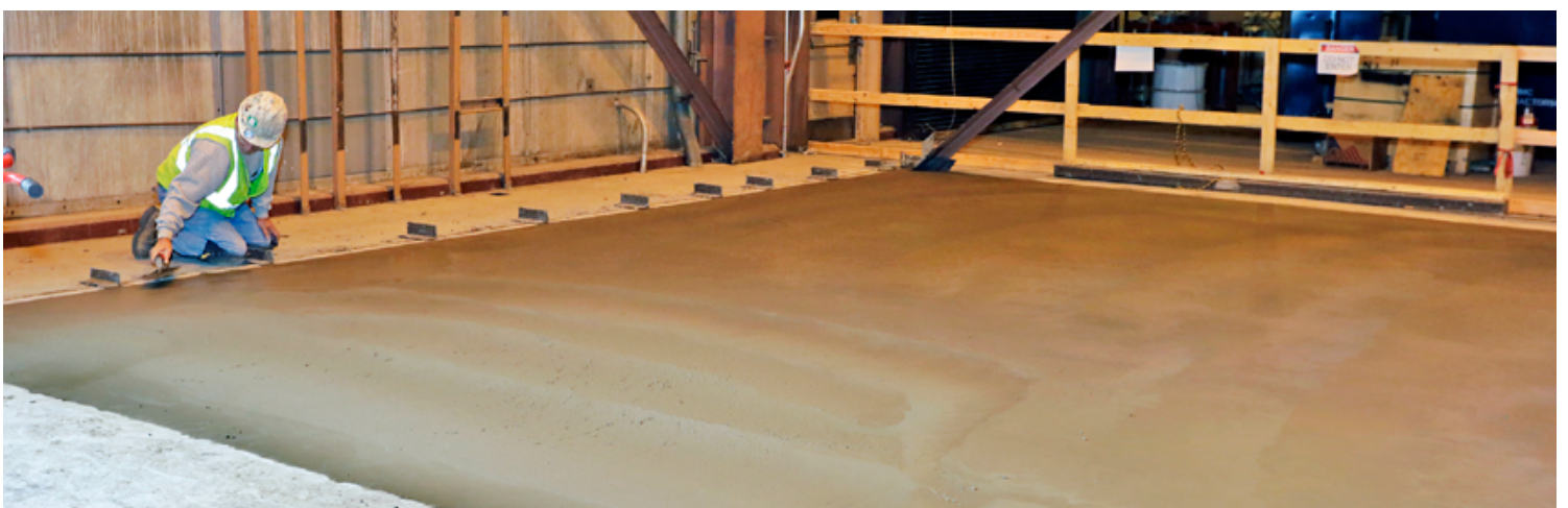
A worker puts the finishing touches on the final quadrant of the cement floor in the C Site-MG Building. (Photo by Elle Starkman)
