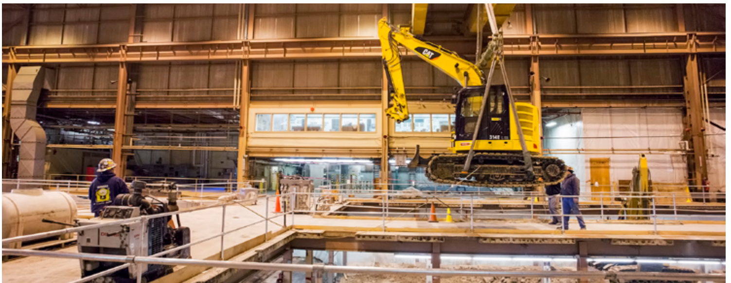
A crane lowers a backhoe into the basement of the C-Site MG Building.
