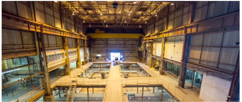
The C-Site MG Building is ready for construction after concrete was removed.
