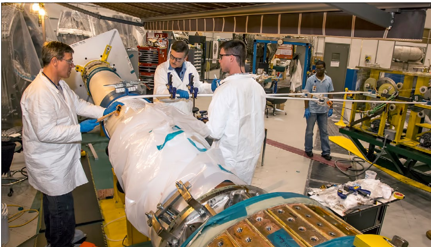
Complex projects like the coil winding of the NSTX-U center stack must go through an extensive work planning and control process that maps out the design, work, schedule, costs and safety plan for the project, all of which must be approved before work begins and updated and approved while the work moves forward. Here technicians work on a coil winding machine that tightly winds two spools of copper conductors onto the center stack.
