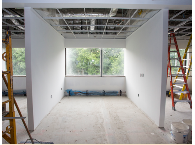
Sheet rock has been installed for future offices in the LSB Building. (Photo by Elle Starkman)
