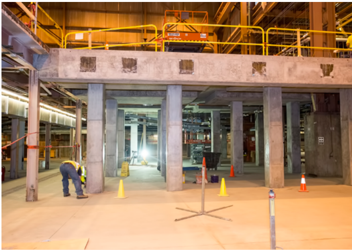
Pillars in the basement of the C Site-MG Building. (Photo by Elle Starkman)
