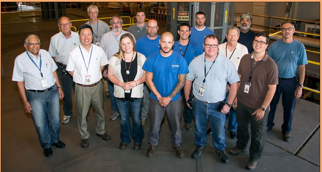
Workers from Voith Hydro completed weld repairs to D-Site Motor Generator No. 1 with strong support from PPPL staffers. Front row from left: Mounir Awad, Chi Man Cheung, Julia Toth, Grant Shue, Tyler Klunk, Morgan Styer; second row from left: Gene Baker, Bill Slavin, Guy Beck, Ben Markle, Harry Krotz, Colin McFarlane; third row from left: Steve Tureikas, Neil Gerrish, Josh Markle, Richard Jones.
