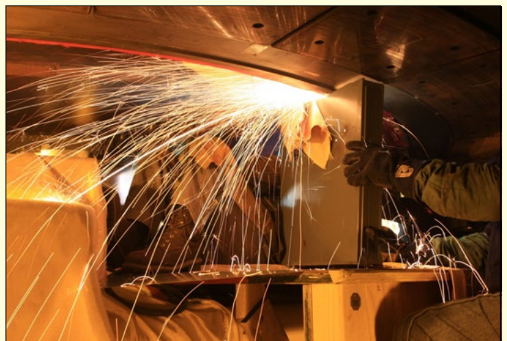
Sparks cascade as a welder assisted by another worker uses an electric arc welder or gouge to remove metal from a defective weld. They are working in a 3-foot space beneath the metal platform called the stiffening ring. The ring in turn is beneath the motor generator. Work on the repair project concluded last month.
