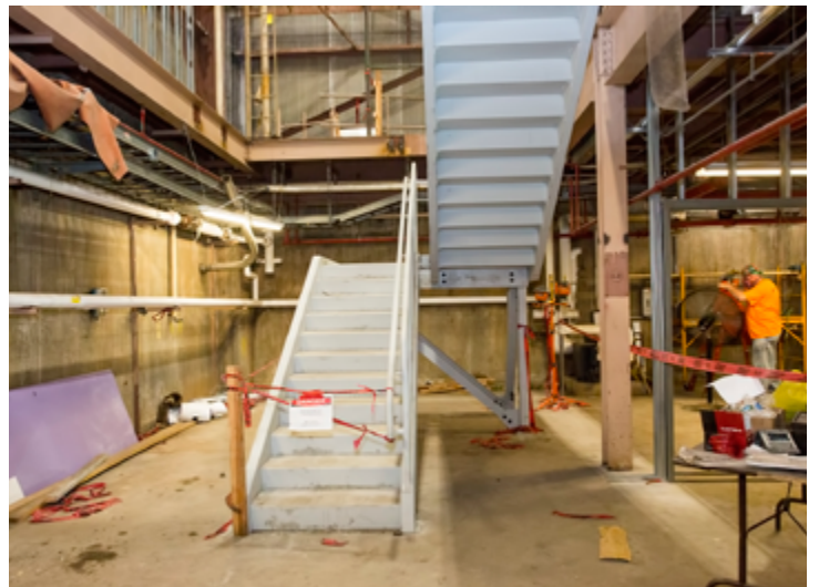
A new stairway in the C Site-MG Building. (Photo by Elle Starkman)
