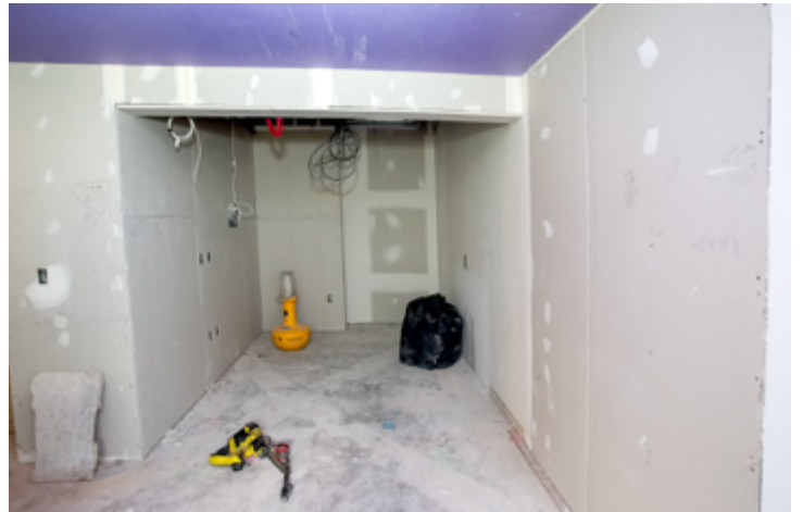
Walls on the second floor of the LSB Annex. (Photo by Elle Starkman)
