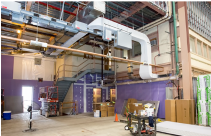
Walls are going up in the C Site-MG Building. (Photo by Elle Starkman)
