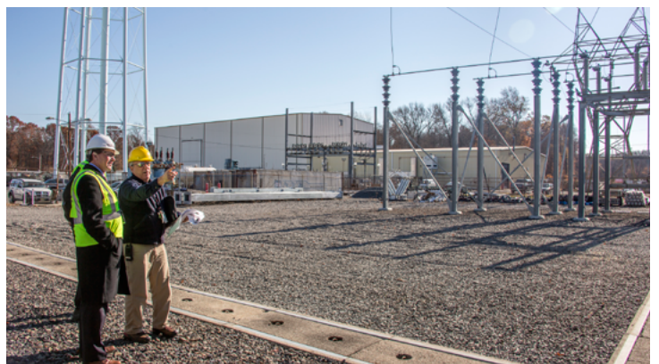
John Lacenere, head of AC Power Engineering, shows McBrearty the power plant. (Photo by Elle Starkman)
