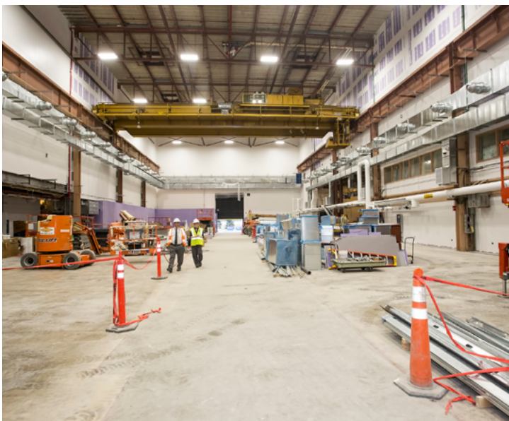
Work on the C Site-MG Building is almost complete. (Photo by Elle Starkman)
