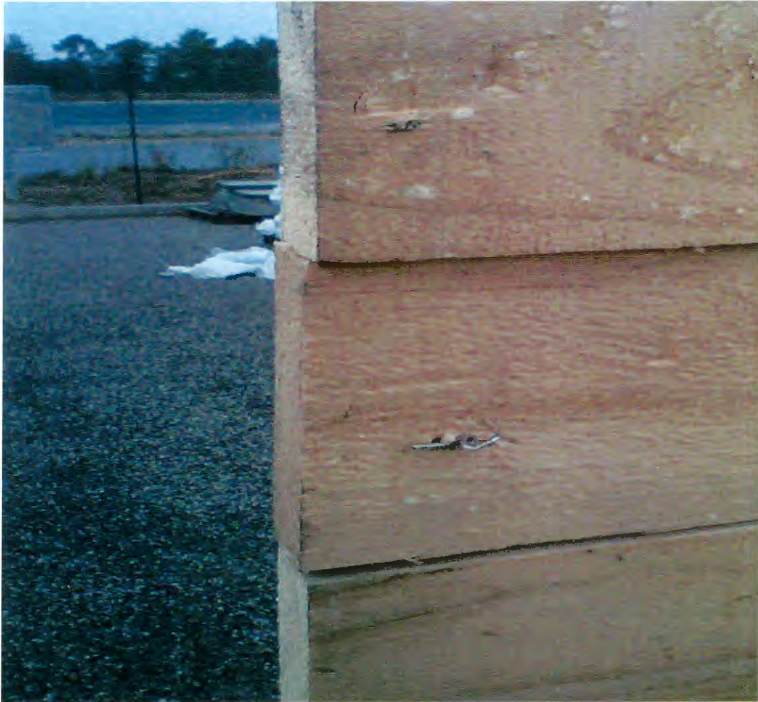
The nails in some covers of the wooden cases failed.
