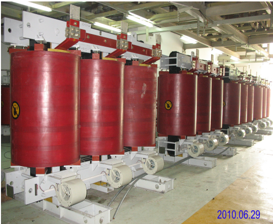
Dry-type converter transformer (2*10/0.815 kV, 6 kVA)
