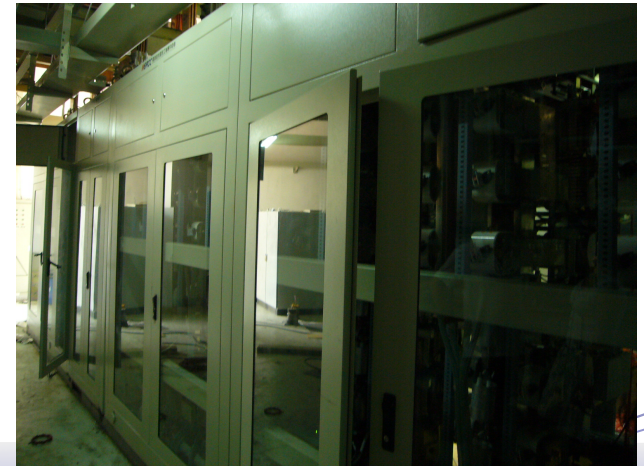
Converter unit (2*1100 V, ±7500A)
