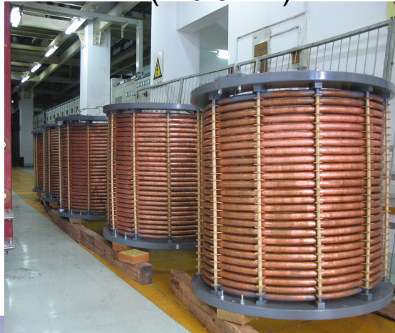
Water-cooling DC inductor (4*0.5 mh)
