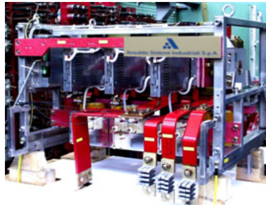
SCB: based on the Static Circuit Breaker design successfully in operation in the RFX-mod toroidal circuit (manufacturer: Ansaldo Sistemi Industriali)
