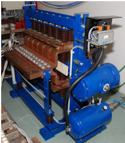
BPS: based on the BPS prototype of FDU of ITER (manufacturer: Siemens)
