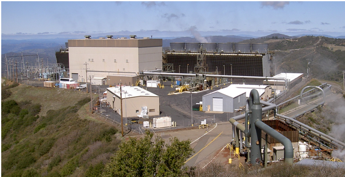
Figure 19 – “Sonoma Calpine 3” at “The Geysers”, the world's largest geothermal field, 22 geothermal power plants, 350 wells, 725MW, located in the Mayacamas Mountains, California, USA
