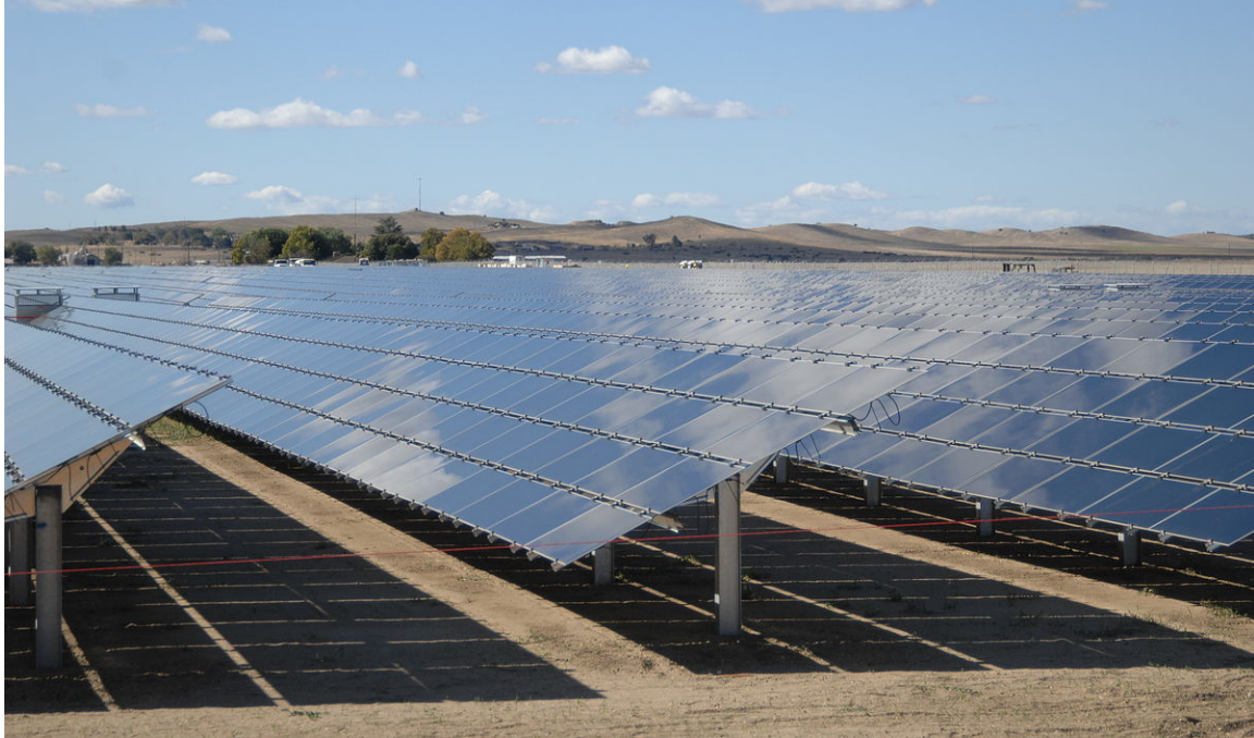
Figure 9 – PV Panels (total of 9 million) at “Topaz”, 550MW (2014), San Luis Obispo County, CA, USA
