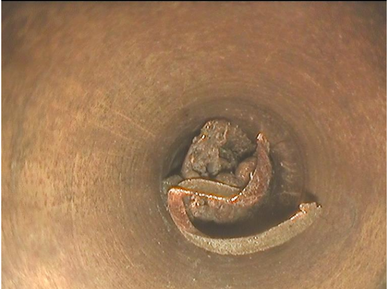
Figure 103 – Braze Joint #3 blockage – view from plane B
