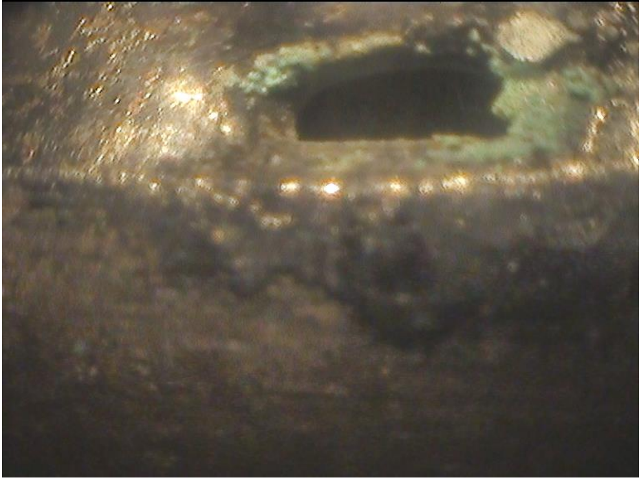
Figure 102 – Braze Joint #2 void – side view
