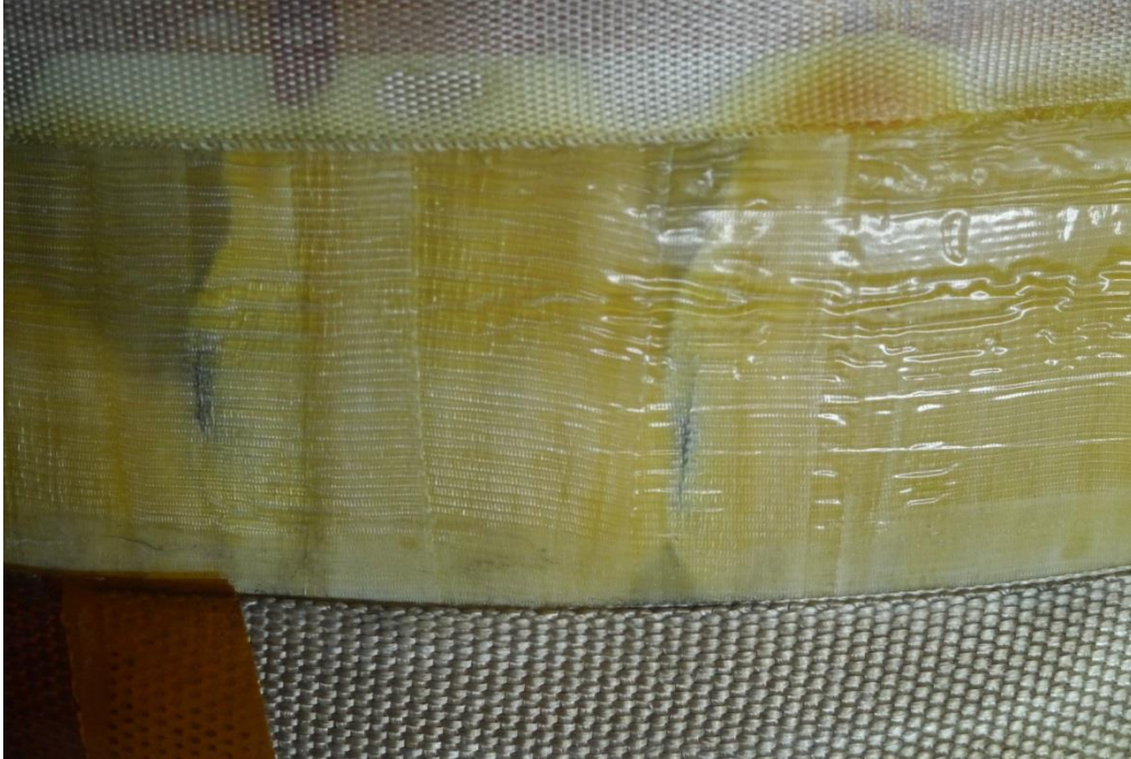
Figure 22 – PF1A-U ground wrap delamination
