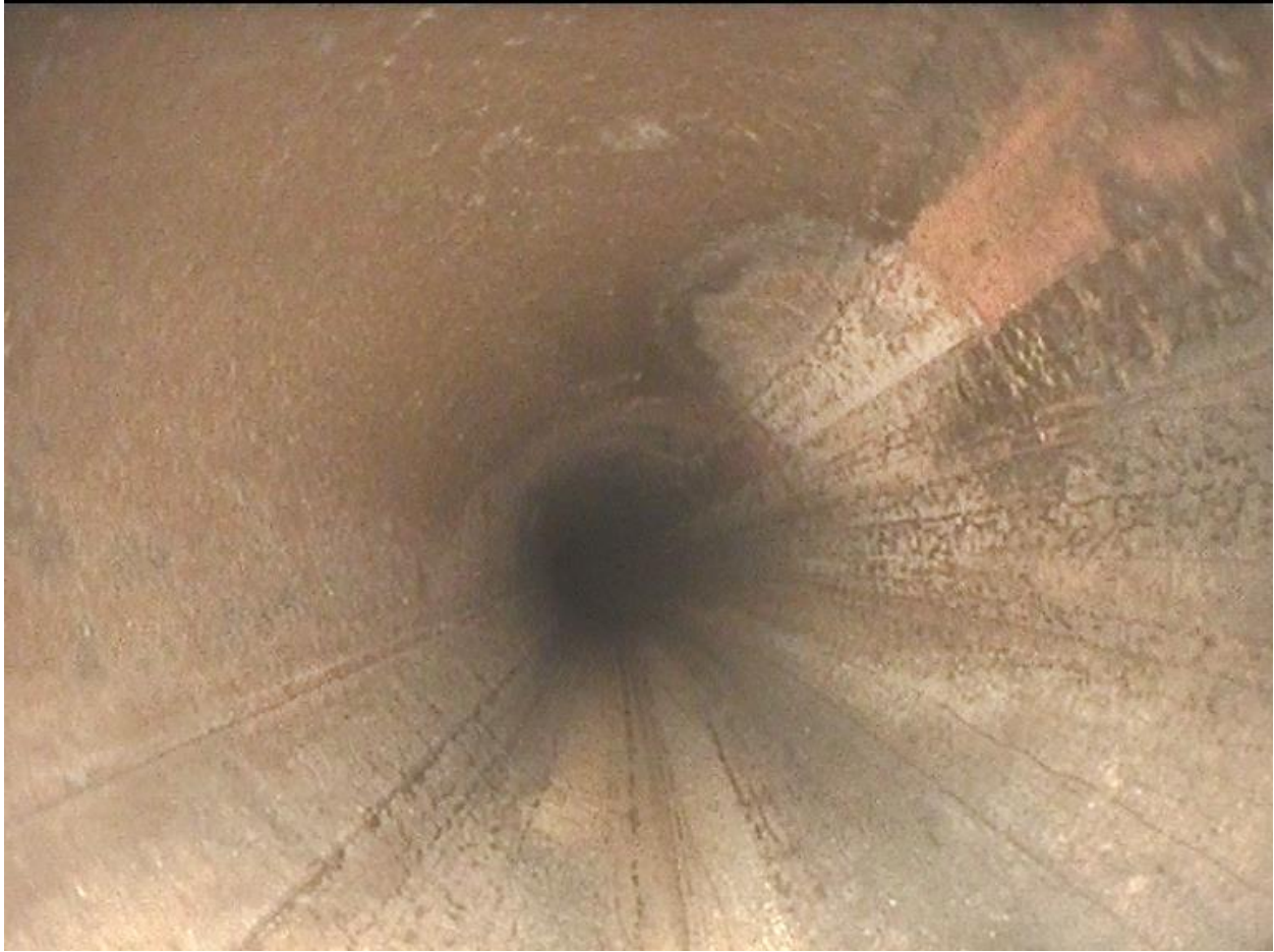
Figure 113 – Discoloration proximal to void in adjacent cooling path
