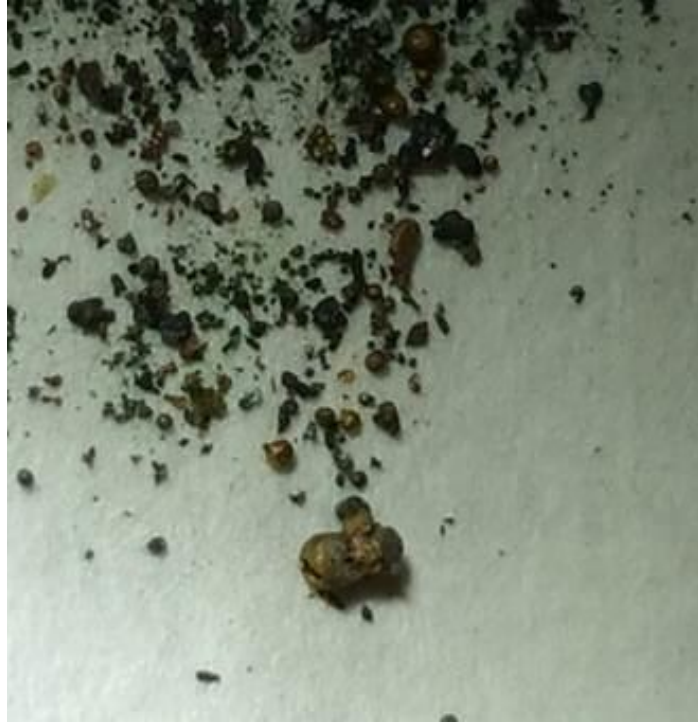
Figure 5 – Debris found in the flushed PF1A-U coolant
