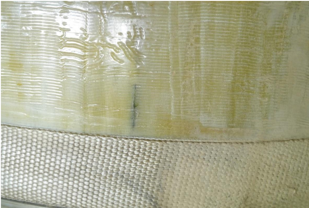
Figure 23 – PF1A-U ground wrap delamination
