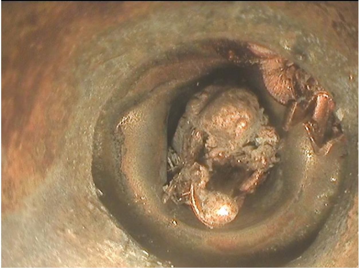
Figure 104 – Braze Joint #3 blockage – view from plane A
