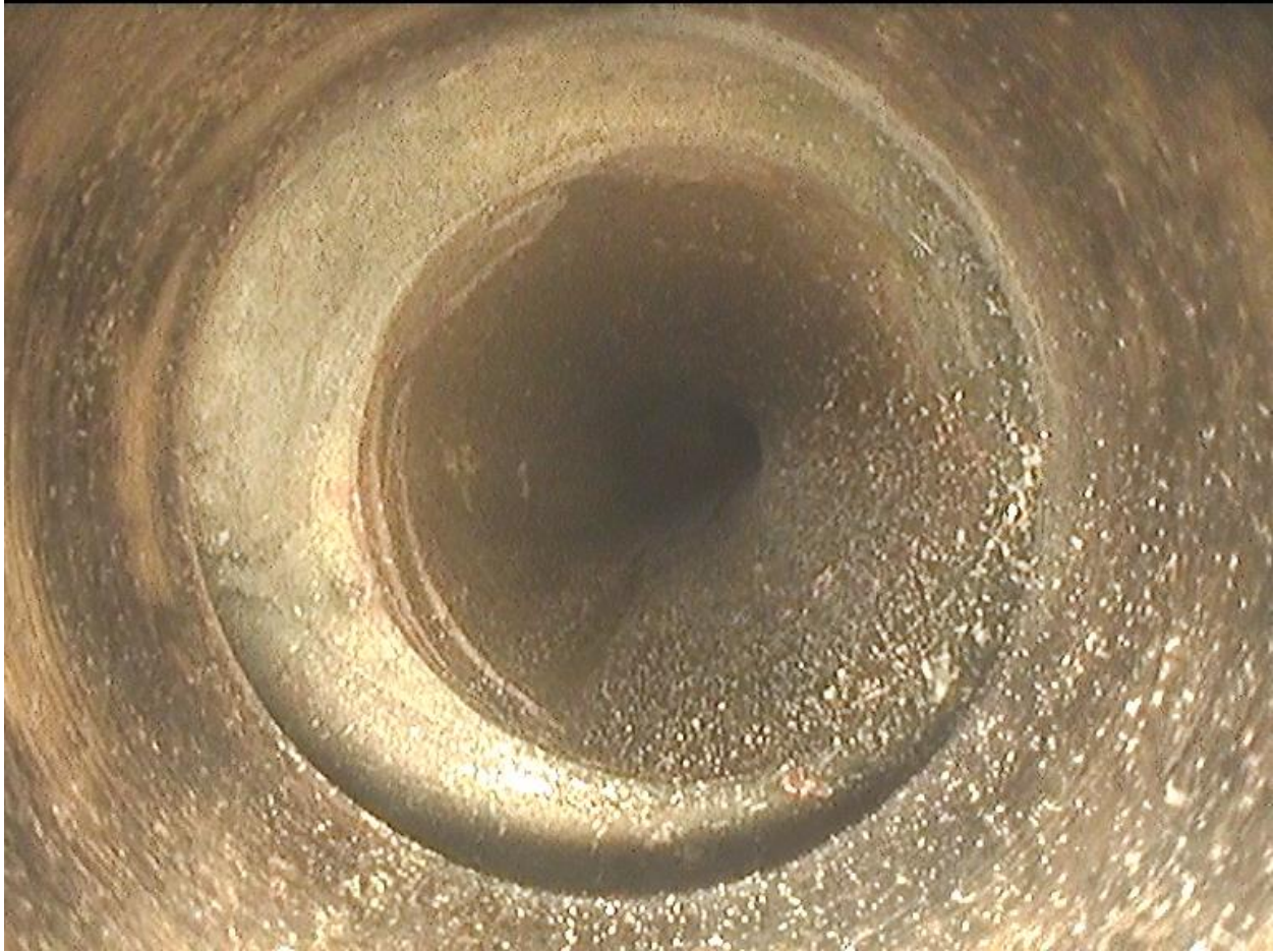
Figure 107 – Braze Joint #4 misalignment – view from plane B
