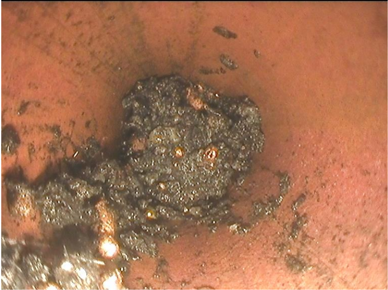
Figure 98 – Braze Joint #1 with blockage – view from plane C
