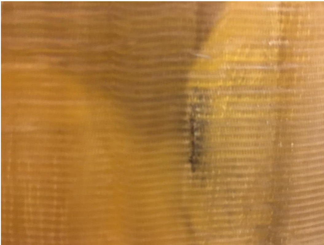
Figure 21 – PF1A-U ground wrap delamination
