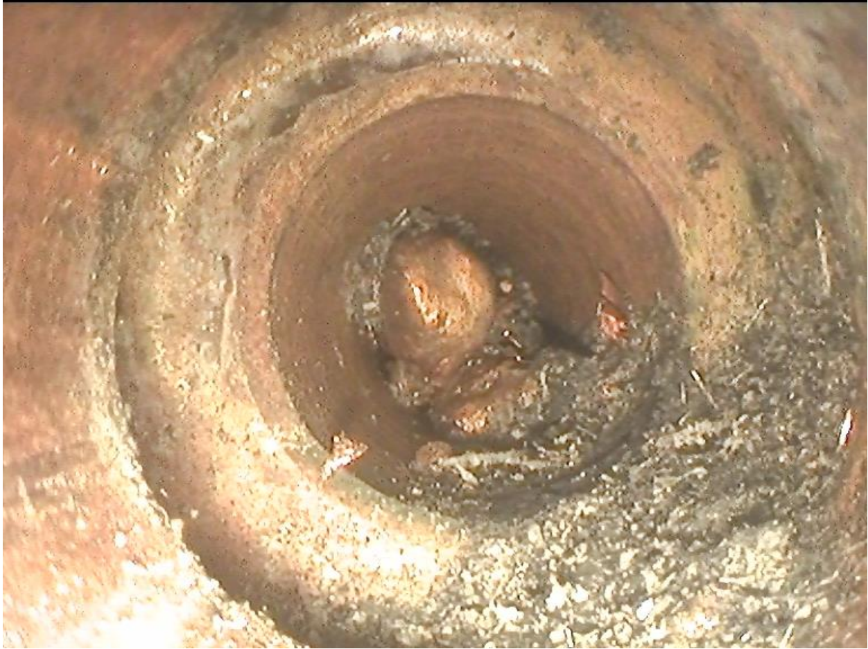
Figure 97 – Braze Joint #1 with blockage – view from plane A
